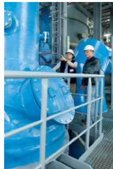
▲ FGDplus demonstration plant at RWE lignite power plant, Niederaussem, Germany
