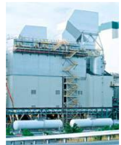
▲ Circulating dry scrubbers (Dry FGD), Virginia, USA
