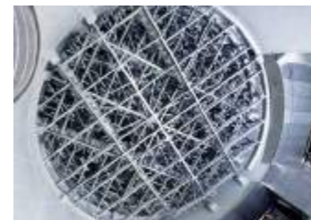
▲ Scrubber at Neurath Power Plant, Germany
