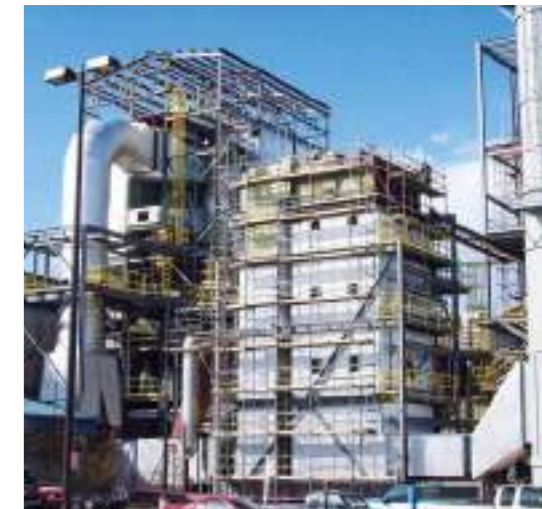
▼ Dry Sorbent Injection and Tail-End SCR, Conyers (GA), Pratt, USA
