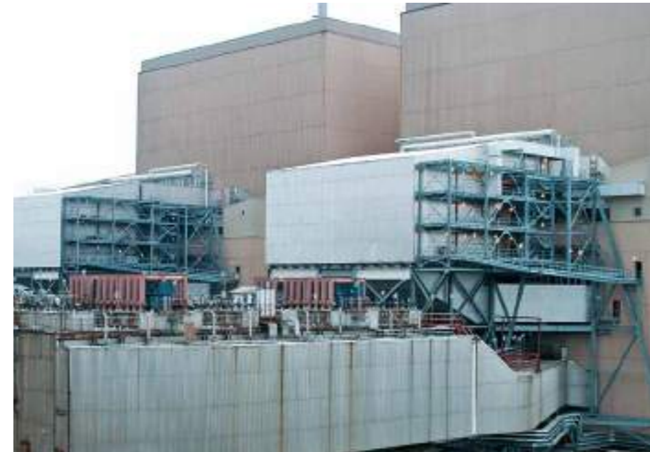
▲ High-dust configuration at Hoosier Energy Merom Power Station, Units 1 & 2, Sullivan (IN), USA
